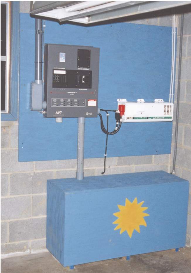
Above: The Ananda Power Center, the Trace inverter, and the vented battery box (with the yellow sun). All these components are safely and neatly installed in Jane's basement
